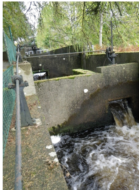
Plate 1b: Original orifices within Sections 6 and 8 – with detector 7 in the background
