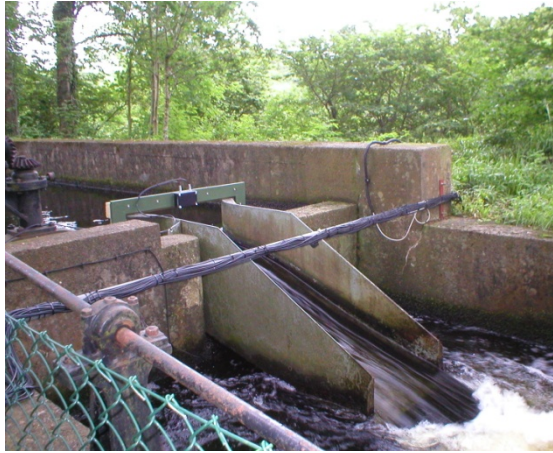
Plate 1c: Section 4 with PIT detector 5 positioned above the resistivity fish counter flume (removed by the 2008 tagging period)
