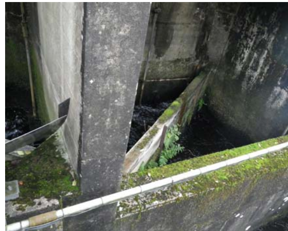
Plate 1f: Section 10 showing diagonal wooden cross walls – all three exits in the dam wall are located within this section
